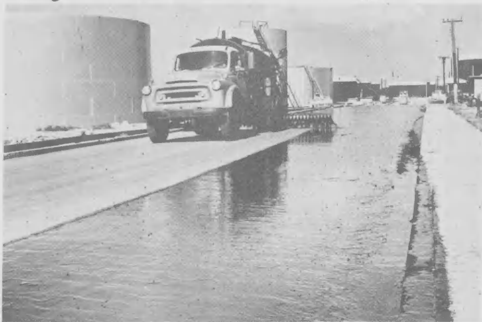
IN LAGO road rejuvenation work a tar truck sprays the roadway with RC-O cutback asphalt. This not only seals the old roadway but acts as a bond for granite chips spread on the oiled surface.
